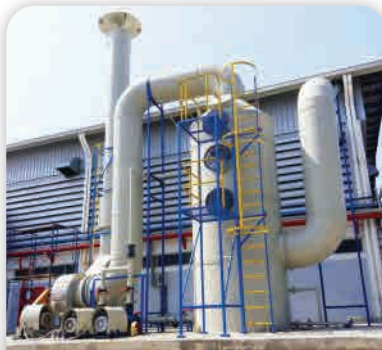
Electronic | WET SCRUBBER
